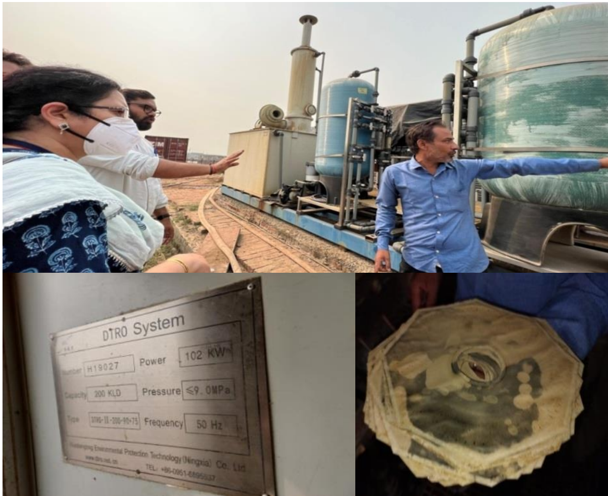
Fig. 8: Visit to DTRO plant and review of Filtration system and its cleaning period and other miscellaneous technical parameters
