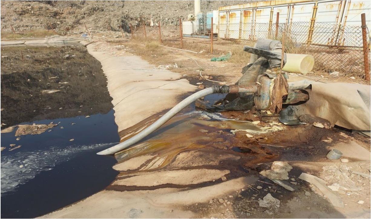
Fig. 10: Reject of DTRO is back into leachate pond
