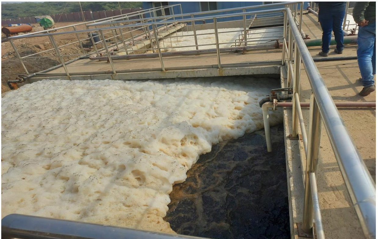
Fig. 7 Dissolved Air Flotation unit
