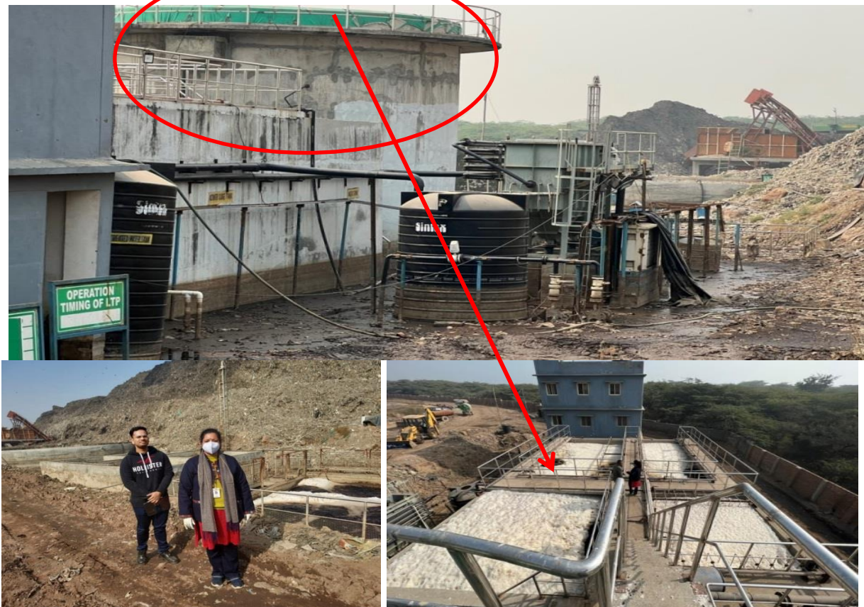
Fig. 6: Leachate treatment plant
