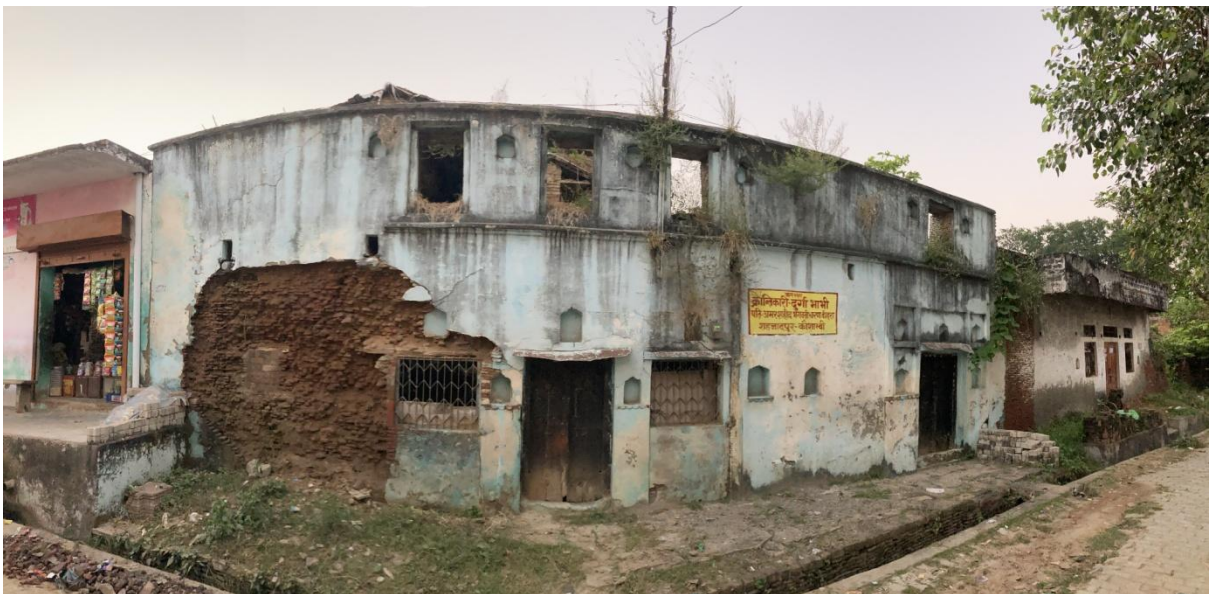
Figure SEQ Figure \* ARABIC 6 Ancestral house of Durga Bhabhi in dilapidated condition, Source: ICH Team, INTACH
