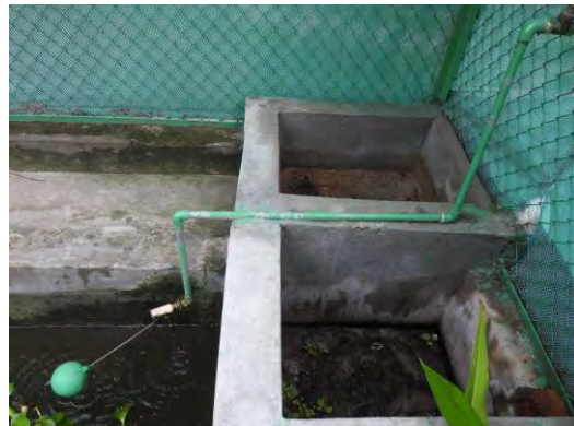
Fig: Filtration Unit of Enclosure II
