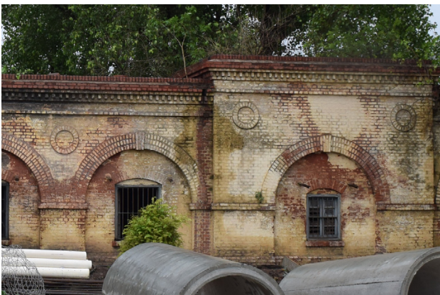
Figure 55 Semi-circular arches with a prominent keystone in colonial buildings. (Source - Primary survey, visited on 18 th August, 2019.)
