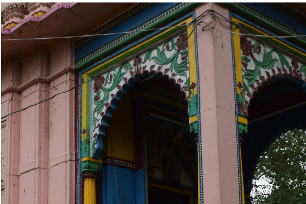
Figure 53 Multi-foliated arches with floral mouldings at a Shiva temple (Source - Primary survey, visited on 18 th August, 2019.)
