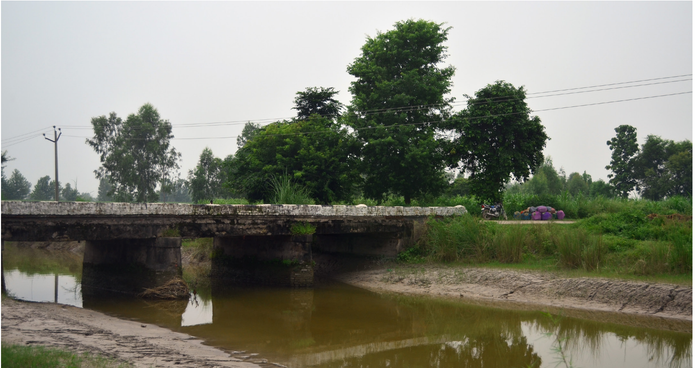
Figure 9 : Bridge over Ganga Canal in Bijnor district. Source: Primary study by AH Division, INTACH Team
