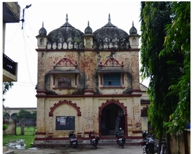
Figure 34 : Entrance to Bijnor Inter College in Bijnor City, also known as Sultana Masjid. Source: Primary study by AH Division, INTACH Team
