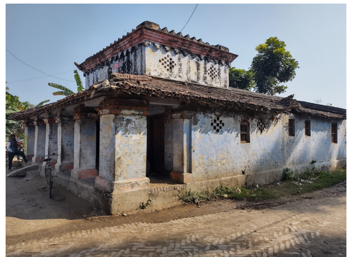
Figure 36: Exterior view of Bhagra Post Office in Mohanpur Source: Primary survey by AH Division, INTACH Team
