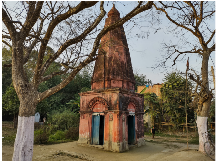
Figure 39: Exterior view of Shiv Mandir at Patori Source : Primary Survey by AH Division, INTACH Team
