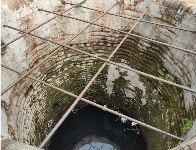
Figure 51: Interior view of well showing the curved surface of the internal wall in Vidyapati Nagar Source : Primary Survey by AH Division, INTACH Team
