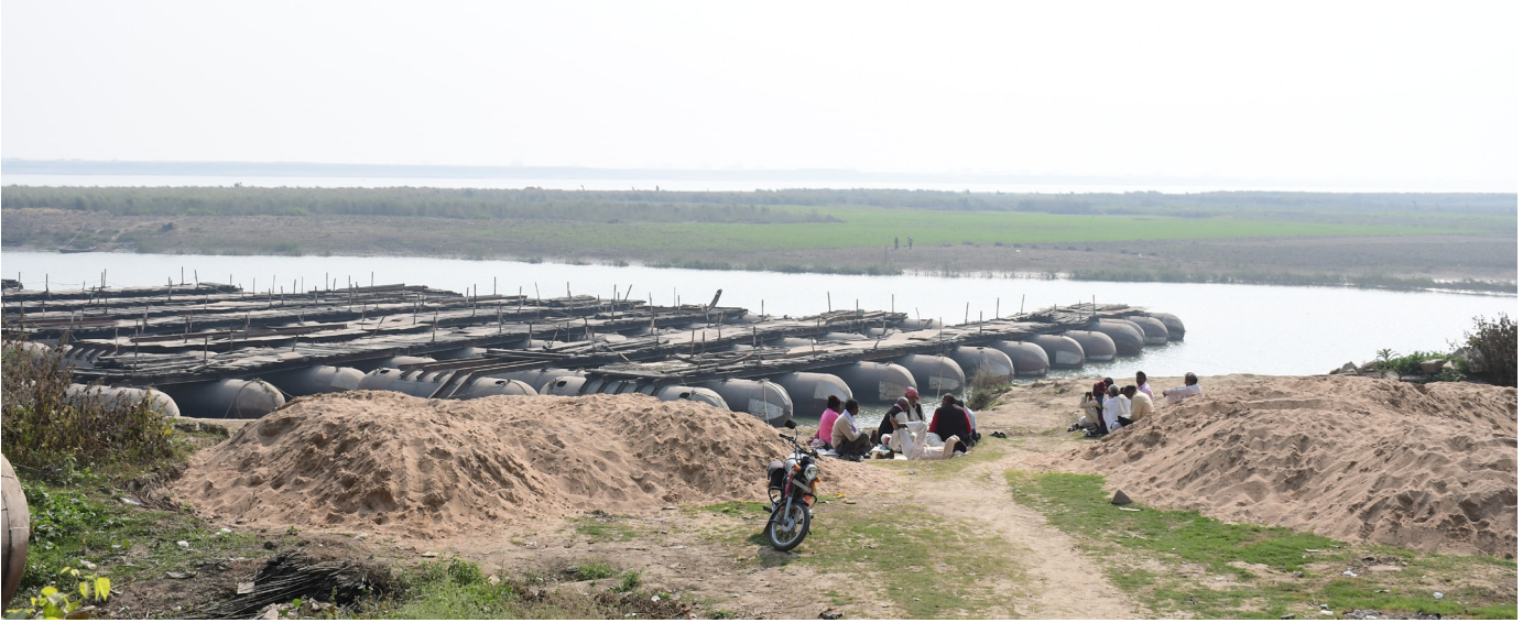
Figure 5 : Incomplete boat bridge connecting Ballia district to Buxar district. Source: Primary study by AH Division, INTACH Team
