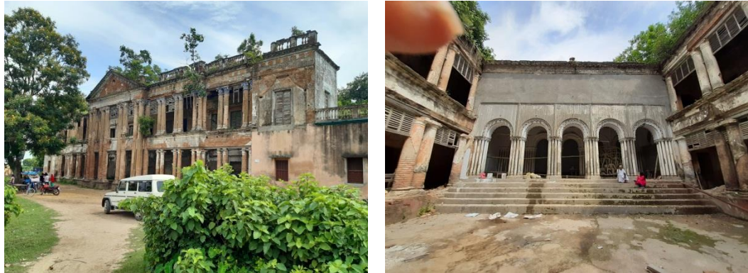
Figure 20 Kunjaghata Rajbari a) Palladian facade and b) Central Courtyard. Source: Personal Visit by INTACH Team
