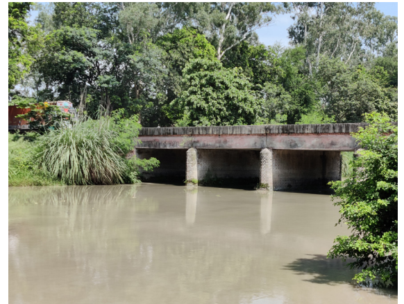
Figure 37: Colonial Bridge, Upper Ganga Canal Source: Primary study by AH Division, INTACH Team
