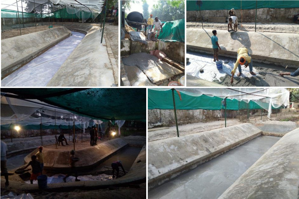
Laying of plastic sheet and concrete mix in the base of the water-body
