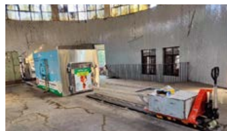
Fig 3: Advanced cremation with provision for performing all rituals and regulating emissions using alternative energy source (electric or LPG/CNG). All photographs courtesy Green Revolution Foundation, New Delhi.
