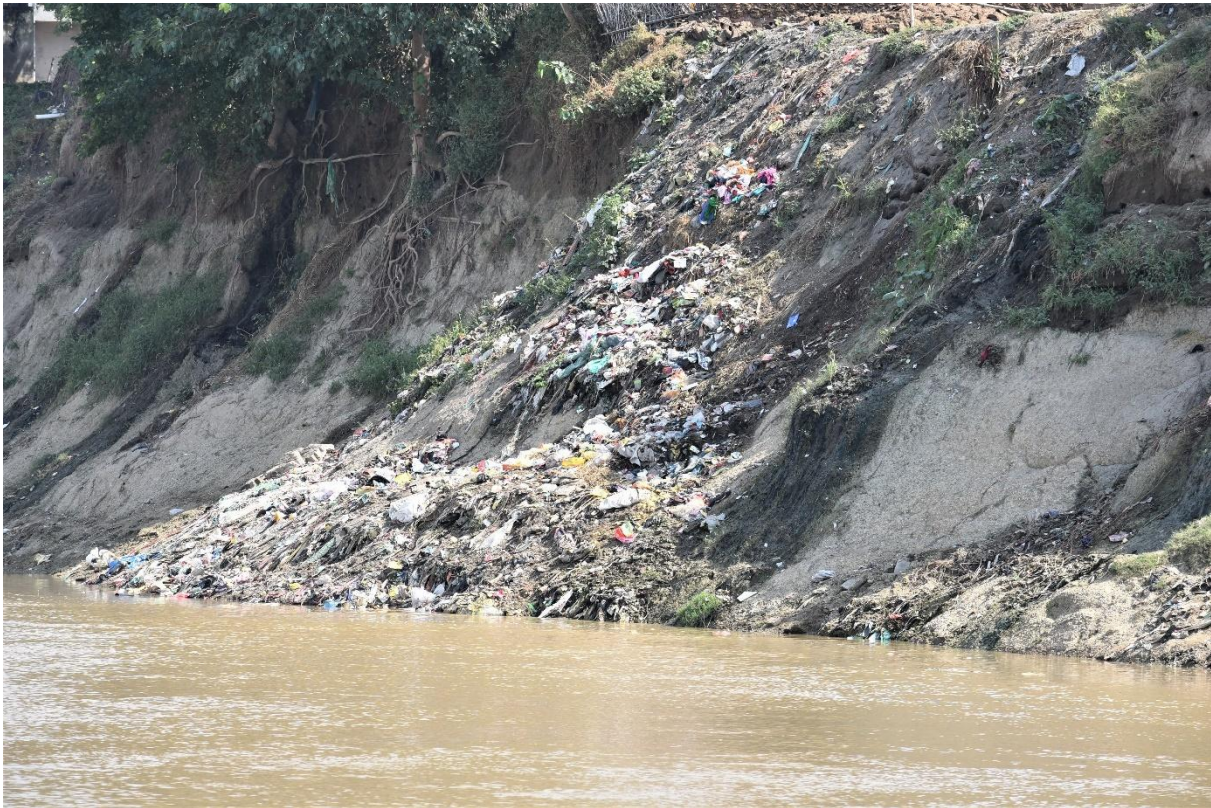
Image 54 : Solid And Liquid Waste Entering Ganga River As Observed Near Bara Village
